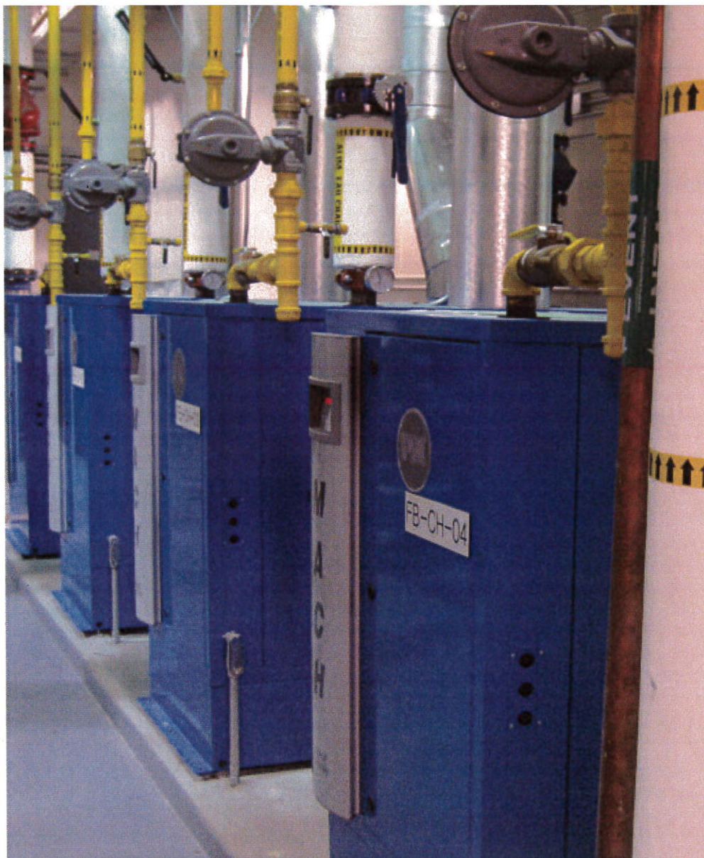
Patterson-Kelley, P-K MACH aluminum condensing boilers treated with TGWT’s tannin for more than three years, installed at a major hospital.
