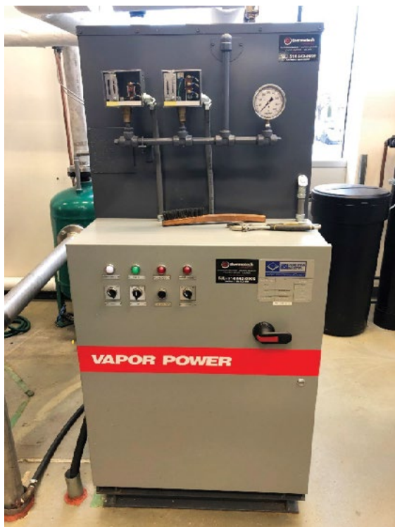
Figure 15: This small electric boiler allowed us to perform simulations. Conditions: 125 to 150 pounds per square inch (psi) (353 to 366°F). Carryover simulations were done using NaCl/NaOH to reach the CCC at a threshold conductivity of 7,000 to 8,000 microsiemens per centimeter ( \mu\text{S}/\text{cm} ) and physically by increase the steam demand. Tannins were effective at a level of 8 ppm in preventing carry-over at the moment of injection as well as after ~20 hours of operation, and beyond conductivities of 10,000 \mu\text{S}/\text{cm} . \text{Ca}^{2+} ions were dosed using a solution of \text{CaCl}_2 .
